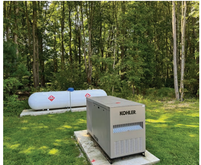
A $30,000 federal grant made possible the purchase of a standby propane back-up generator to ensure continuity of electrical power at Village Hall and police headquarters.
